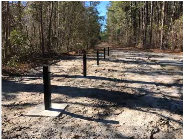
Sumter County, near airport 5 wells
