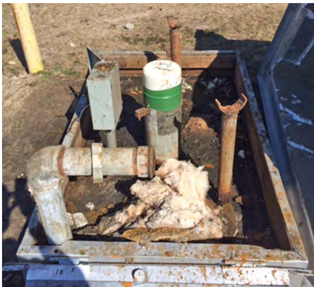
Figure 20. Unused supply well AIK-0344 at Oakwood-Windsor Elementary School in Aiken County. The well is 404 feet deep well and is screened in the Crouch Branch aquifer.
