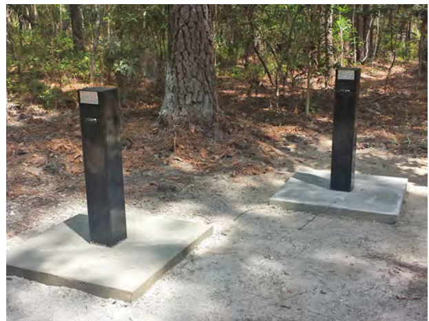
Figure 18. New monitoring wells at Hobcaw Barony in Georgetown County. GEO-0387 (left) is screened in the Gordon aquifer (95 feet deep) and GEO-0386 (right) is screened in the surficial aquifer (39 feet deep).
