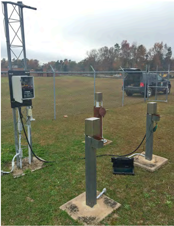
Figure 15. Real-time data system installation in Orangeburg County (ORG-0431).
