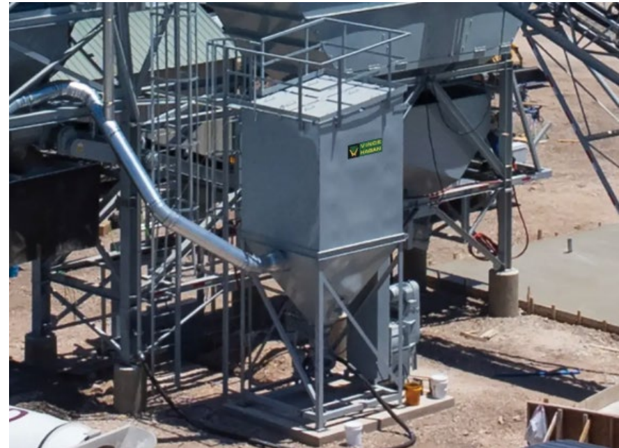
Central Dust Collector
