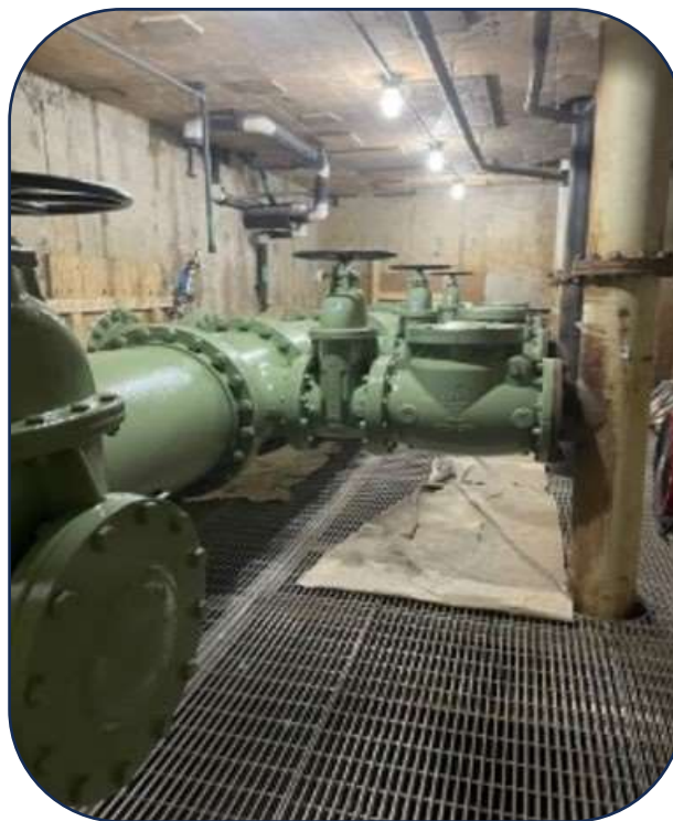
New raw water pumping manifold at the Chester Metropolitan District water treatment facility. (Photo provided by RIA.)
