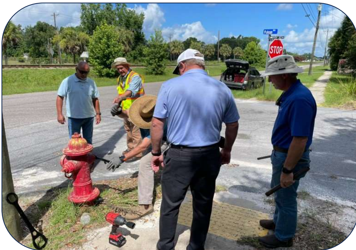
SCRWA staff work with operators in the Town of Allendale to maintain non-operational fire hydrants. (Photo provided by SCRWA, June 2025)
