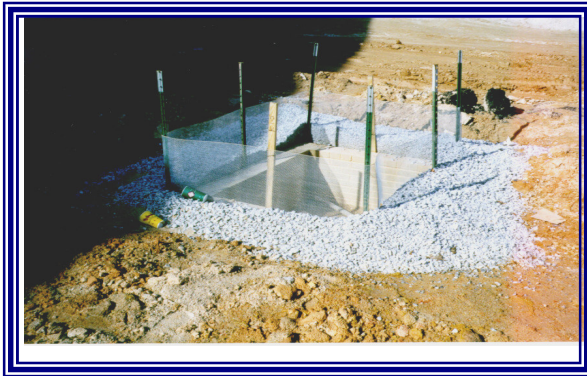
Hardware Fabric and Stone Inlet Protection
