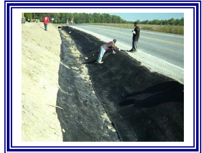
TRM Channel Application
