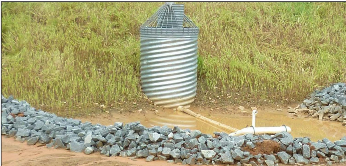
Photo: Principle Spillway's Riser Structure with Skimmer
