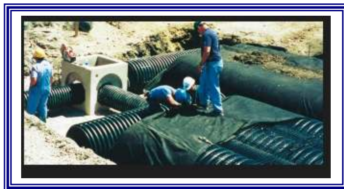
HDPE Underground Detention
