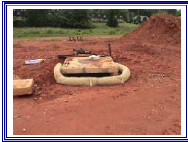
Sediment Tube Inlet Protection
