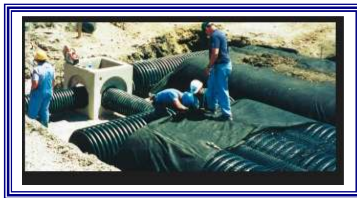
HDPE Underground Detention
