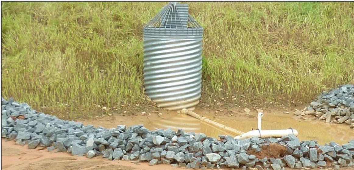
Photo: Principle Spillway's Riser Structure with Skimmer
