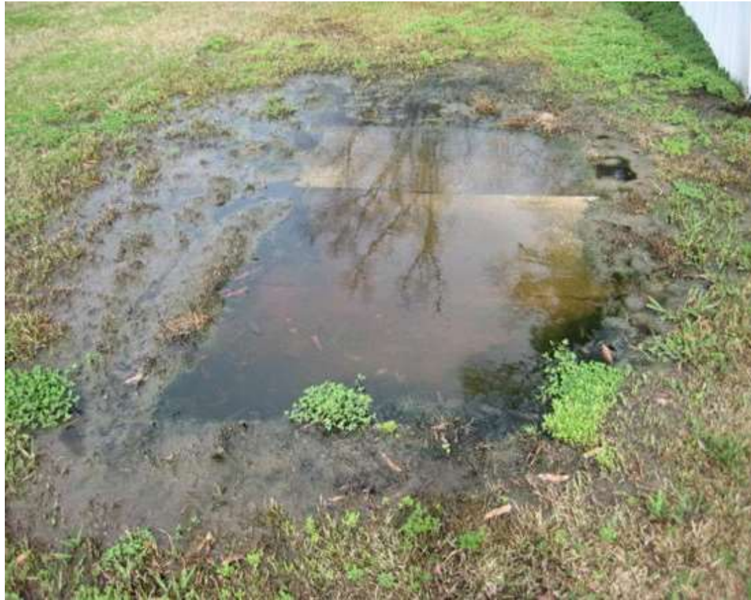
Figure 3. Sewage pooling on a residential property due to a malfunctioning septic system
