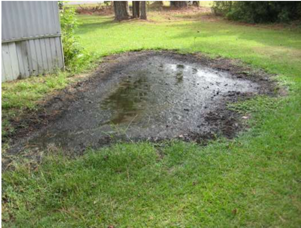
Figure 4. Sewage pooling on a residential property due to a malfunctioning septic system
