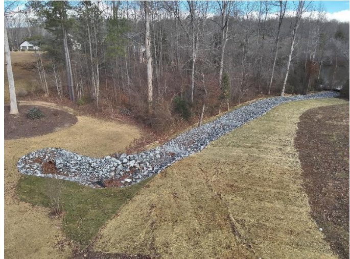
Stormwater outfall improvement
