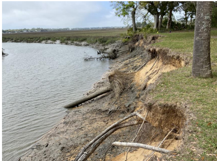
Bank erosion at the proposed project site
