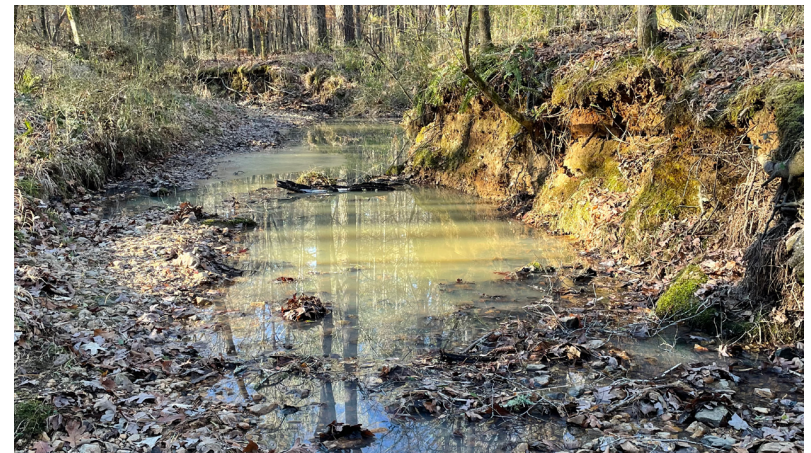
An eroded streambank.
