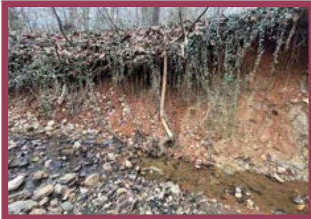
Figure 1.28 Eroded Stream Bank (City of Fort Mill)
