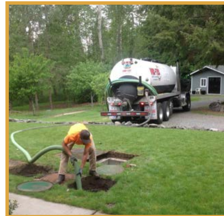
Figure 3.8 A septic system pump out (Vac-Tec Septic & Water LLC)
