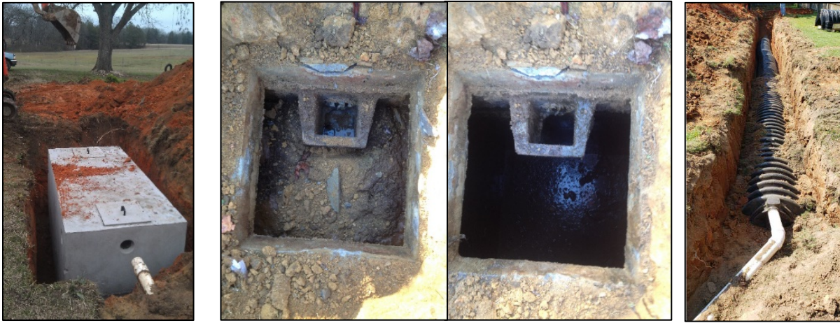
Examples of a Septic Tank Replacement, Before and After Maintenance, and Drainline
