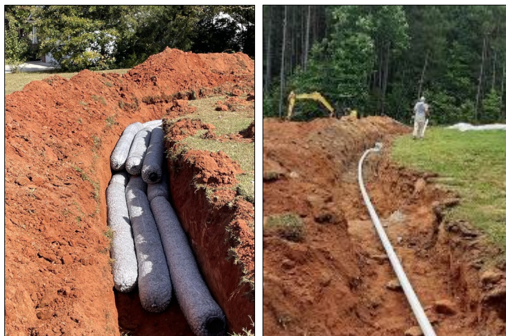
Septic drain-line repairs in the Three & Twenty Creek Watershed. EZ-flow pipe (left), outlet pipe (right).
