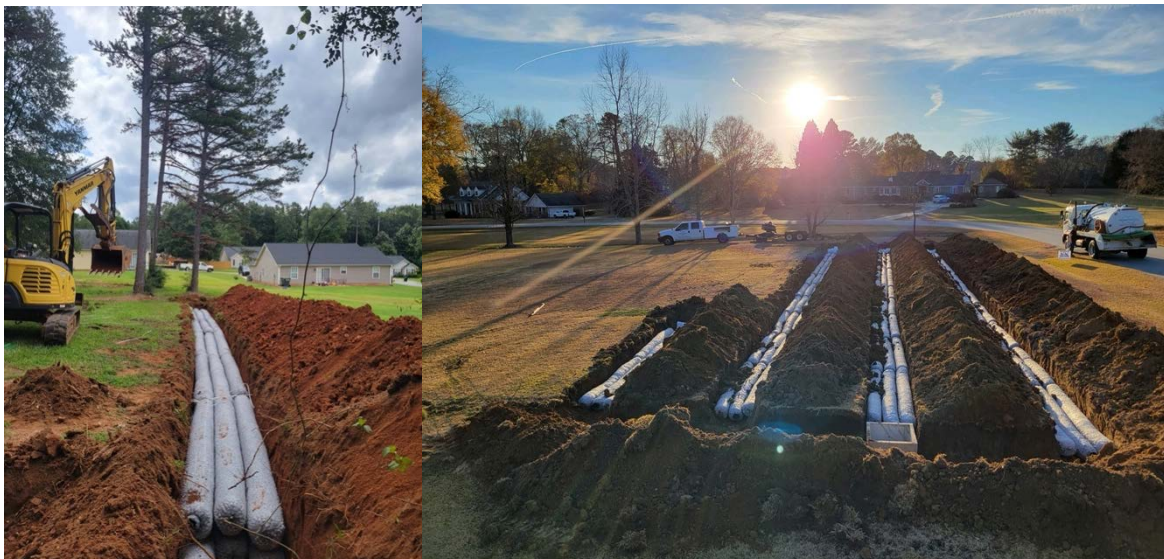
Fig. 35. Examples of septic repair work in the Three and Twenty Creek watershed, which neighbors the Twelvemile River watershed. (photo provided by Upstate Forever).
