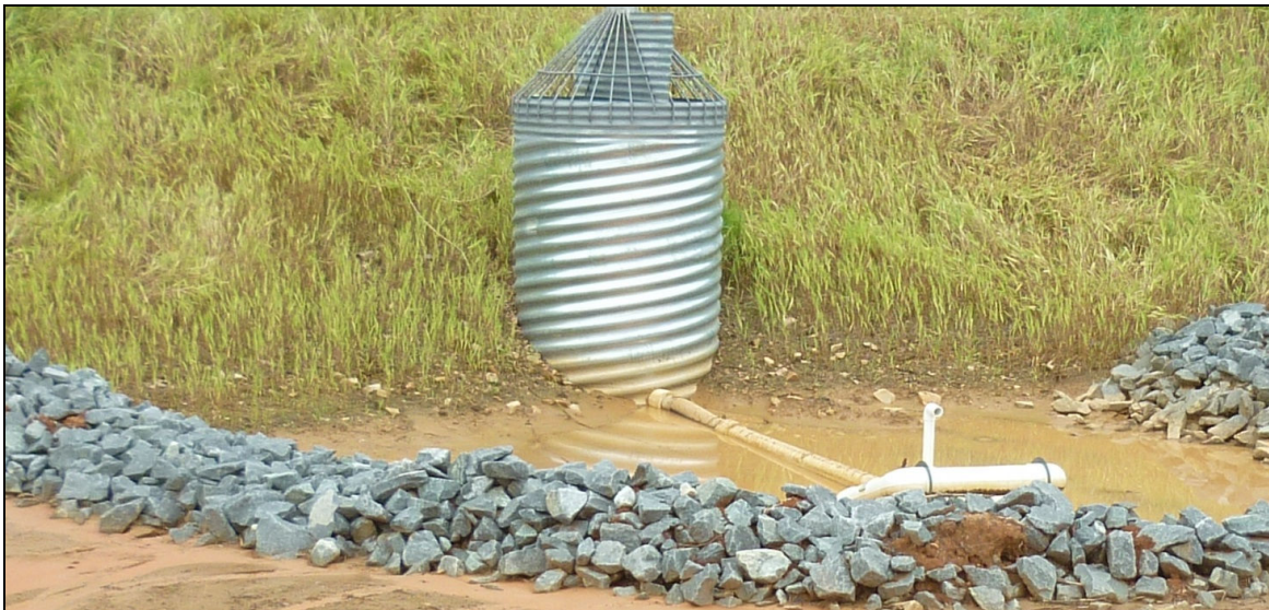
Photo: Principle Spillway's Riser Structure with Skimmer
