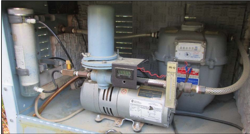
Inside View of Air Monitoring Station
