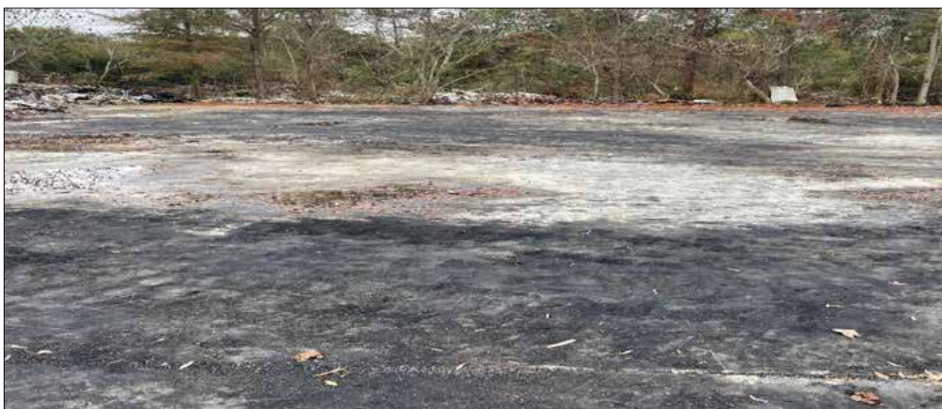
Views of the Trebie Road Site before and after removal operations in FY24. Most of the hazardous substances were stored in the containers with much of the rest of the site covered by solid waste.
