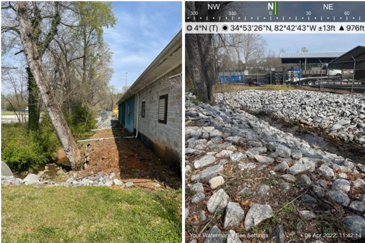
Fig. 42. Disconnecting impervious surfaces from direct discharge to waterways is a critical stormwater pollution prevention strategy. Within these tight quarters shown in the top left image, a solution may be found to do just that as part of a larger park renovation and stream restoration plan. Restoring the tributary to a more natural state will also benefit pollutant attenuation, in comparison to the existing armoring at the tributary.
