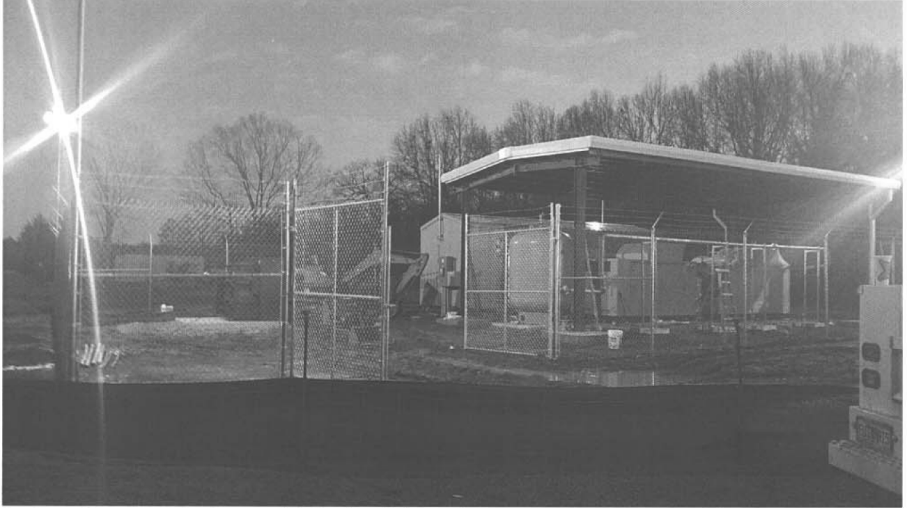
Equipment compound entrance with fencing, lights, and gates
