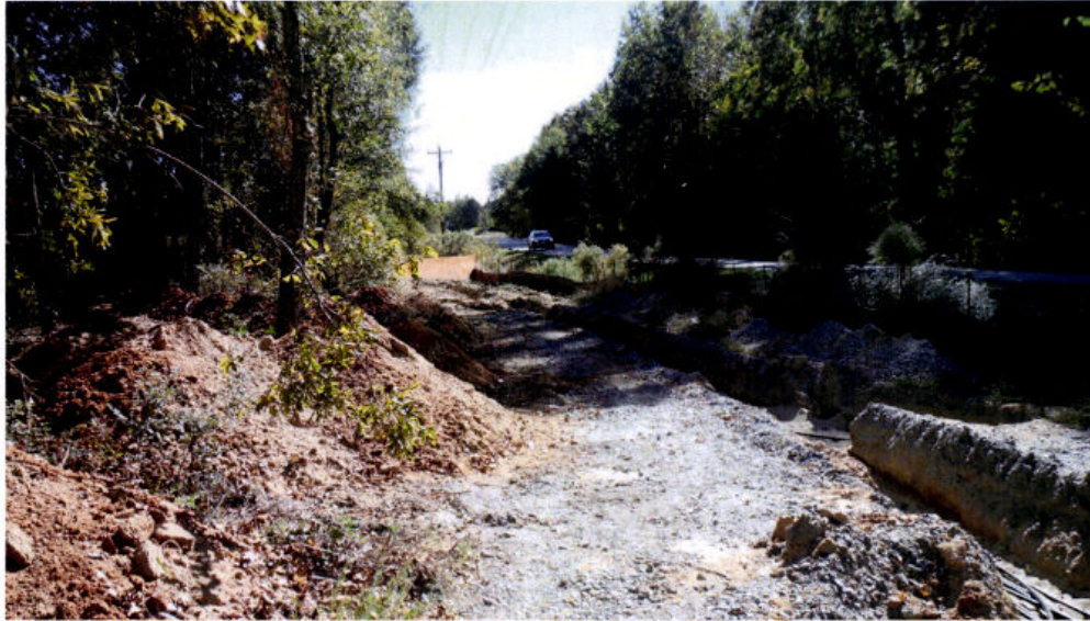
10/21/2016: View of the Cupboard Creek vertical sparging network with West Calhoun in the background. High-density polyethylene (HDPE) piping conveys the compressed air to the sparging wells. Trenches are backfilled with clean fill after pressure testing and tracer wire installation is complete.
