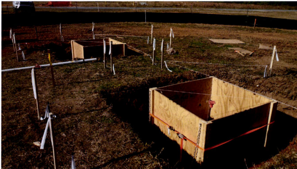
10/31/2016: Aligning the canopy footer forms in preparation for the concrete pour. The canopy will cover the exterior equipment which will be the primary process elements to remediate the site.
