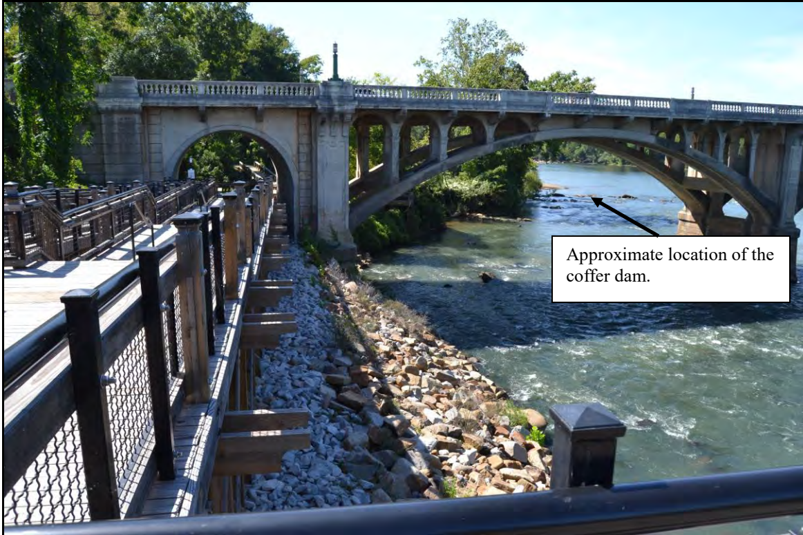
Figure 23. View from Columbia Canal Hydro Plant to project area. Note rip rap.
