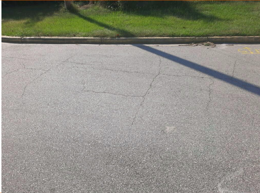
Photo 3: Block cracking near Boring B-3
