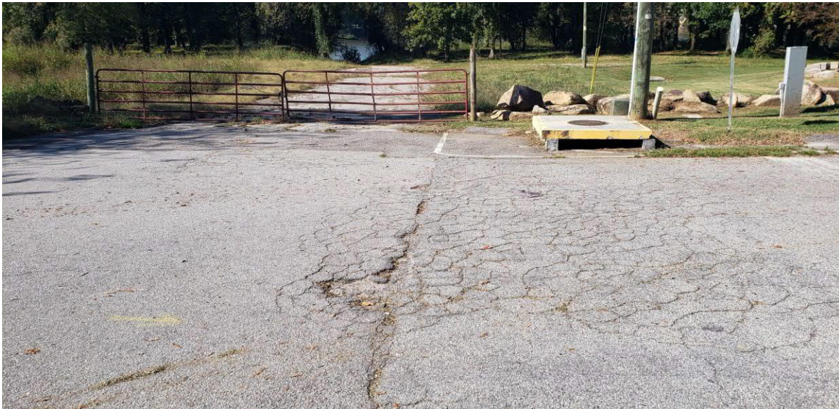
Photo 4: Alligator cracking near Boring B-5
