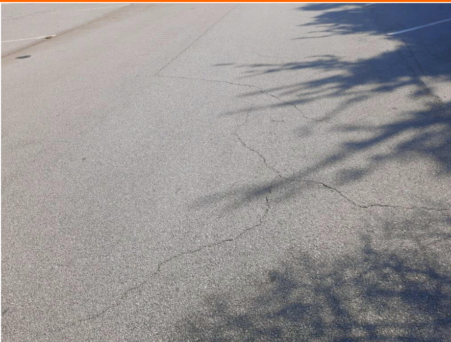
Photo 2: Longitudinal/Transverse cracks near Boring B-2
