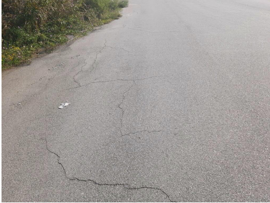
Photo 1: Longitudinal/Transverse cracks near Boring B-1
