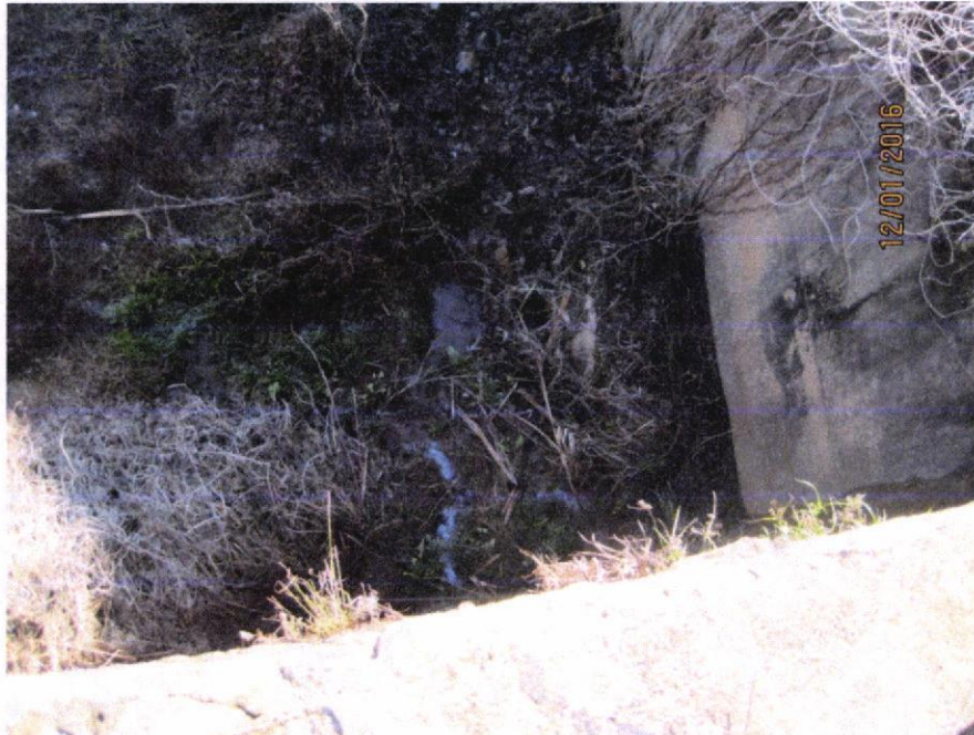
5. Seepage flows along the right toe
