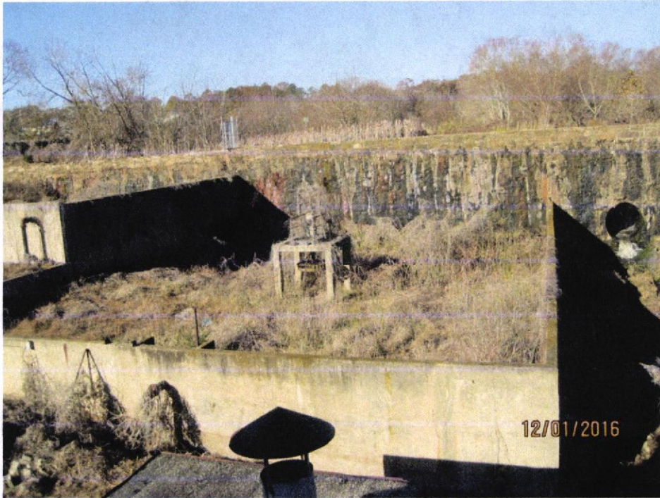
3. Seepage and ochre present on the right face of the dam
