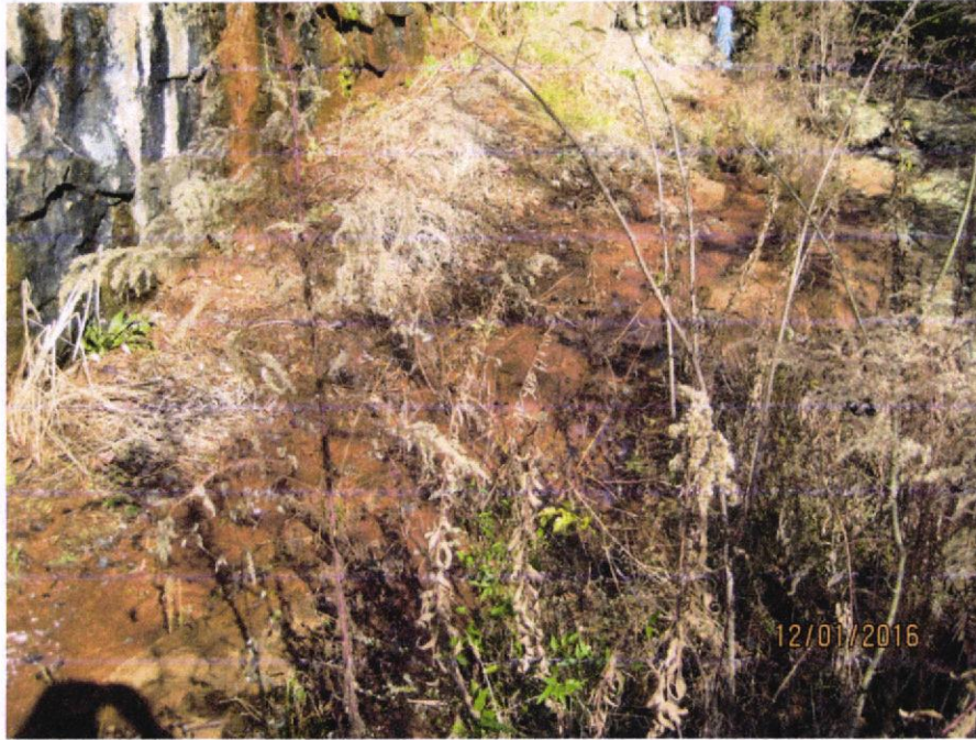
9. Seepage flows along the left toe of the dam
