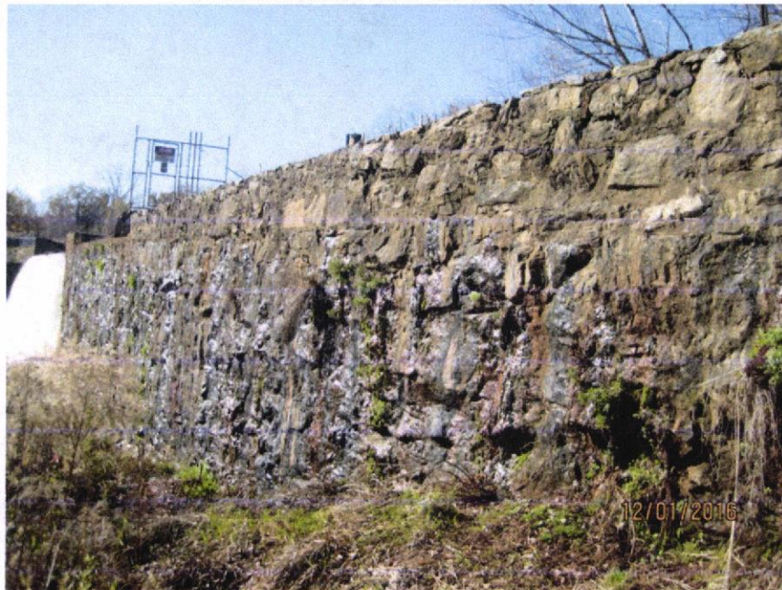
8. Seepage and ochre present on the left face
