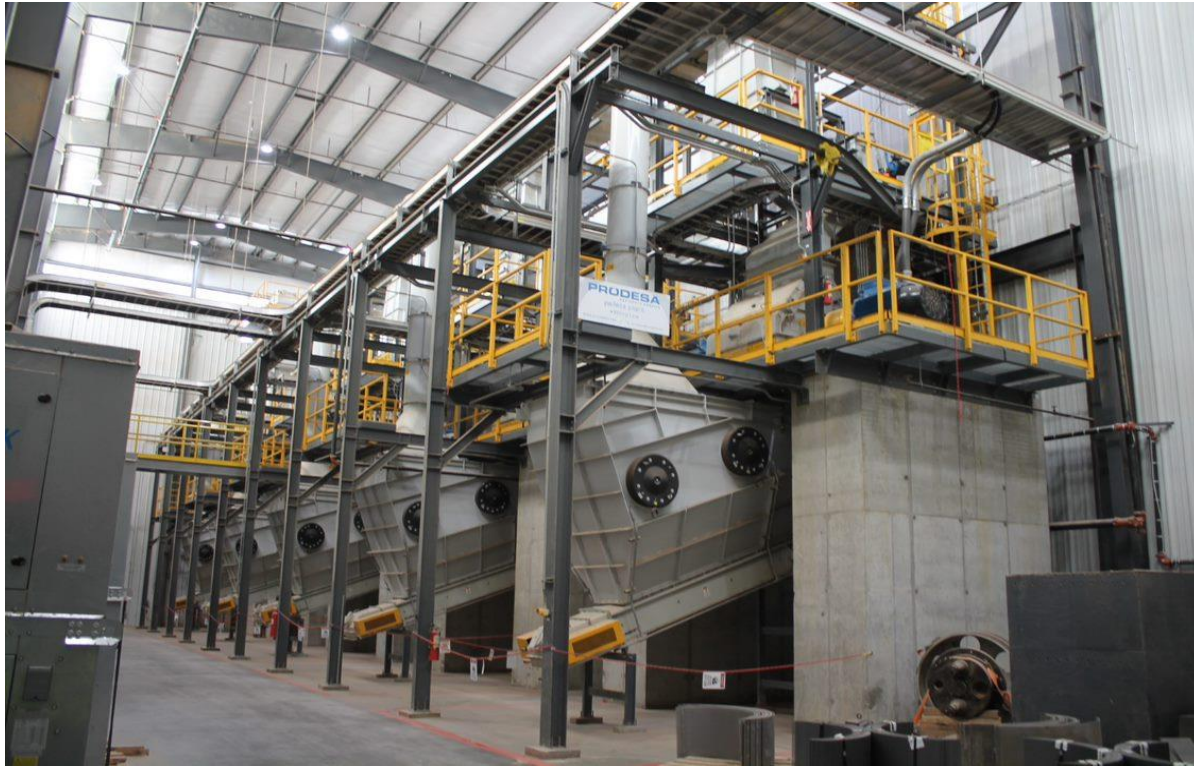
Example of horizontal dry hammermills (existing)
