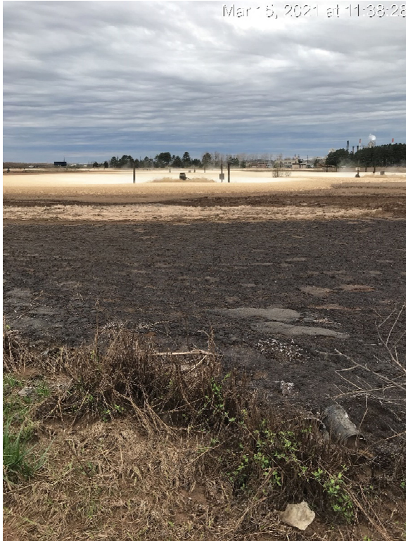
Photo ID: 5 Date/Time: 3/15/2021; 1138 Description: Aeration basin with foam layer
