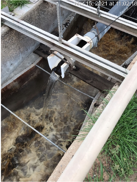
Photo ID: 3 Date/Time: 3/15/2021; 1102 Description: Clarifier decant and sanitary waste
