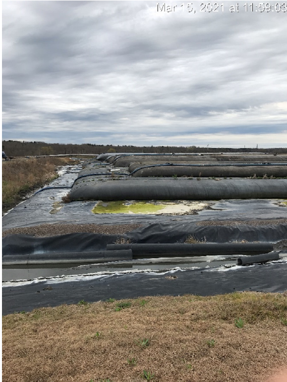
Photo ID: 7 Date/Time: 3/15/2021; 1159 Description: Geotube sludge dewatering system
