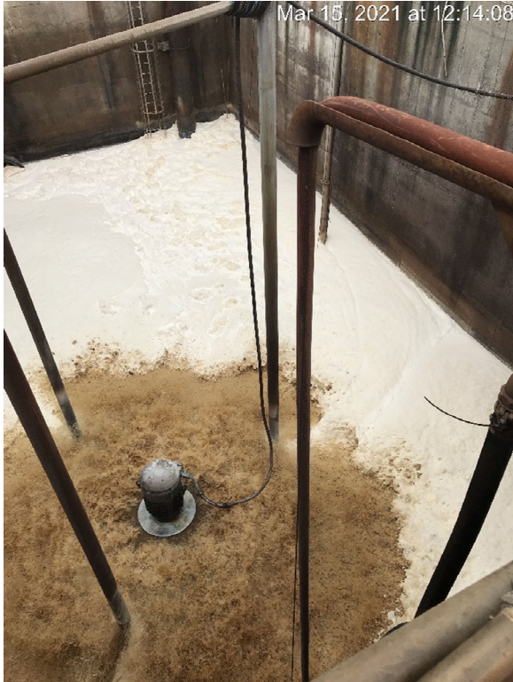
Photo ID: 9 Date/Time: 3/15/2021; 1214 Description: Post-aeration basin
