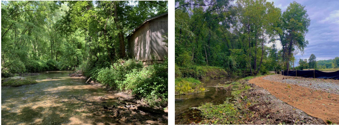
Dover property before photo (left) showing eroded bank and dilapidated building and after (right) hydroseeded and matted bank area
