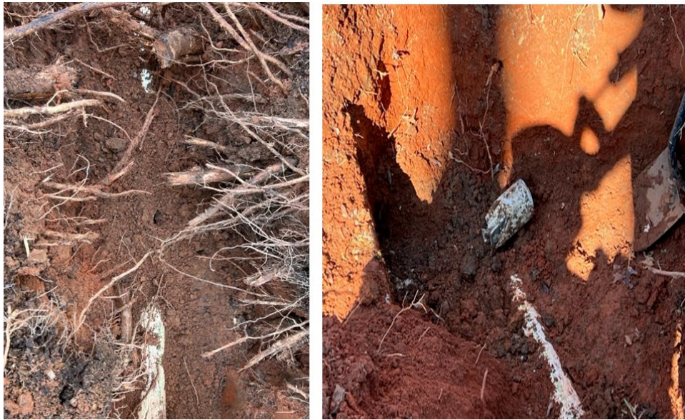
Drain line impacted by roots (left) and visible sludge (right) at elbow of pipe before repair
