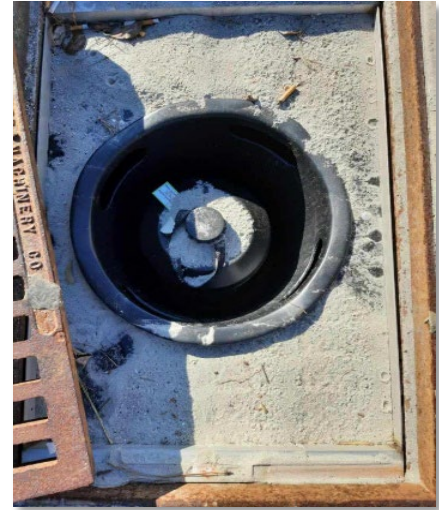
Filtrex Stormwater Catchment Basin Filter on Ocean Blvd
