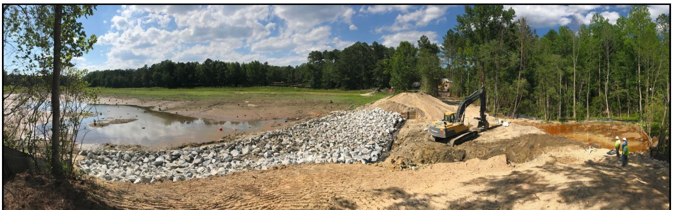
DHEC's contractor breaching an unsafe dam to eliminate risk to downstream areas
