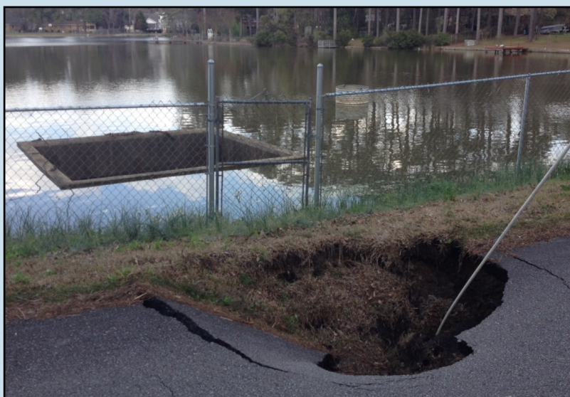
Sinkhole that appeared, and then quickly grew in size, in a public road on a dam in Richland County
